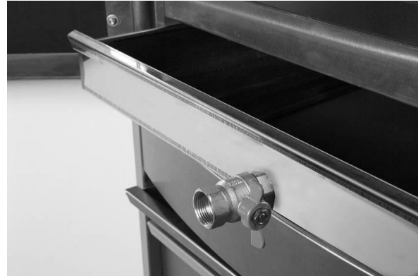
Drain valve closed. (Handle vertically)
